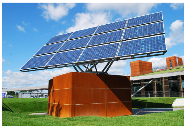
Fig. 9. Solar electric charging station at the SOLON Headquarter in Berlin.
