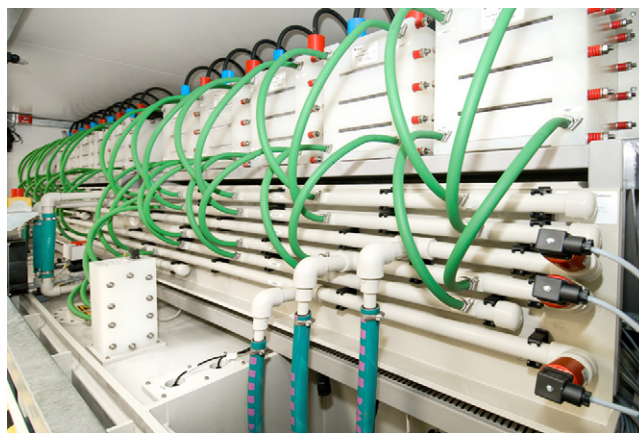
Fig. 1. Cellcube FB 10/100 overall design showing fluid lines and power stacks.
